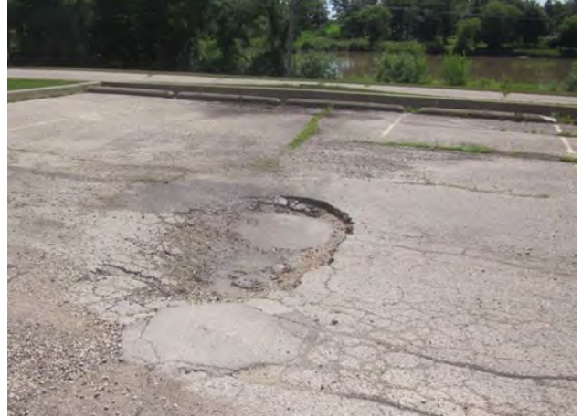
Large pothole in parking lot
