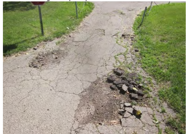
Asphalt path conditions near clubhouse
