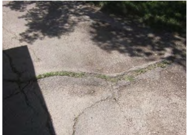
Tree root damage to asphalt paths at clubhouse
